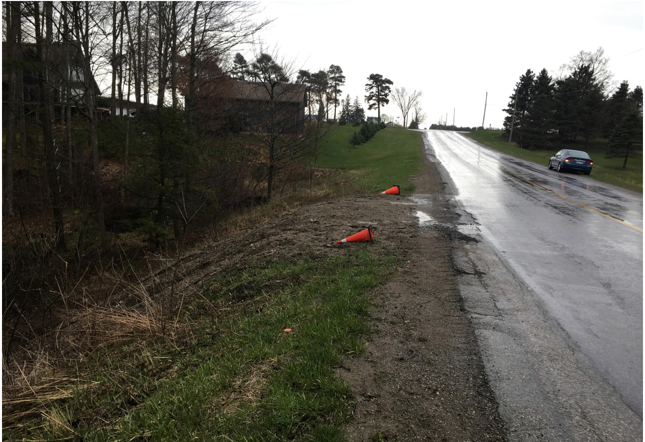
(Above) Carter Road – Facing south. Washout fill marked by temporary orange cones at Mun No 8403. Vertical curve at Chalet Line intersection.
