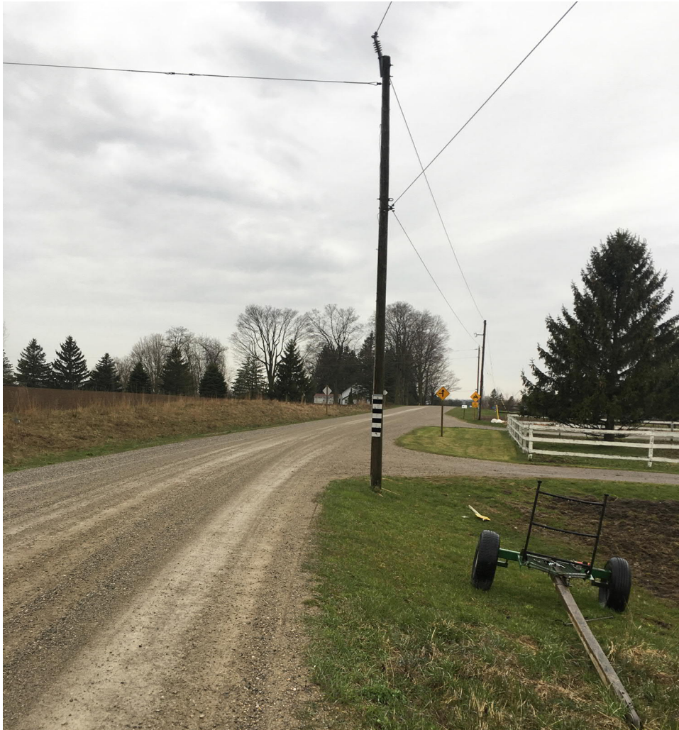
Chalet Line – faded hazard sign and hydro pole in clear zone at Mun No 52220.
