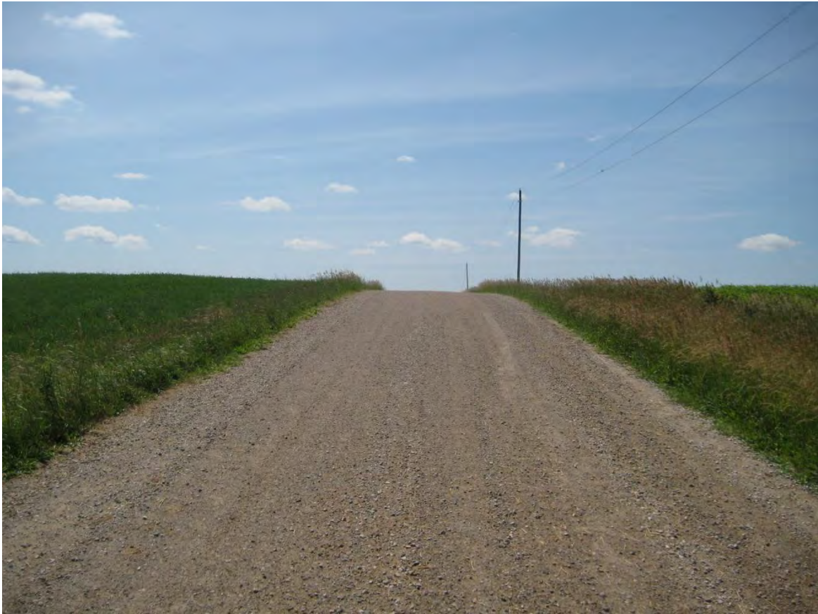
Corless Road – Poor visibility approaching Wilson Line intersection due to vertical alignment.
