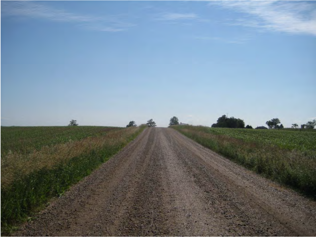
Crossley Hunter Line – Poor visibility approaching Pigram intersection (facing east) due to vertical alignment.
