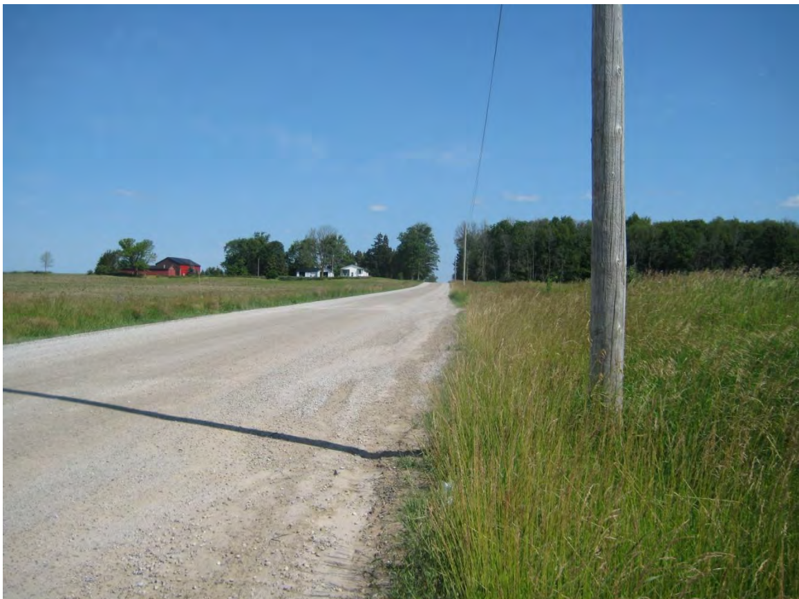
Pigram Line – Hydro poles within clear zone north of Lyons Line intersection, on east side.
