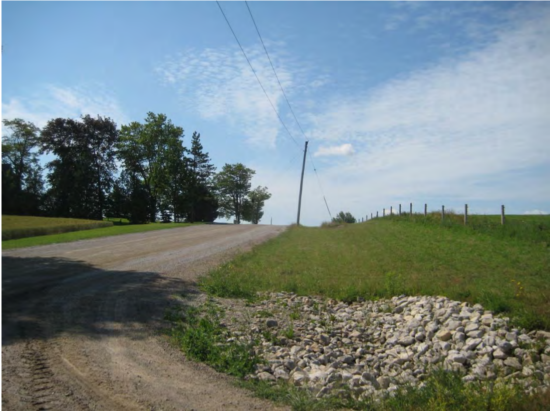
Crossley Hunter Line – Poor visibility on Pigram intersection facing south, due to vertical alignment.
