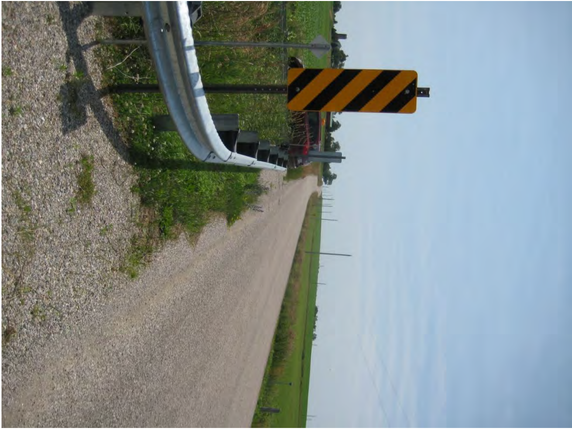
Whittaker Road – Guardrail over Catfish Creek on east side within 1m of roadway.
