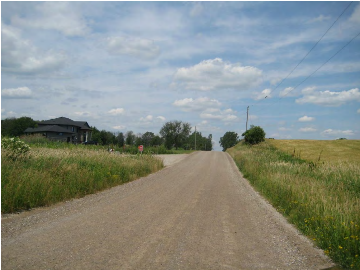
Whittaker Road – Poor visibility due to vertical alignment.
