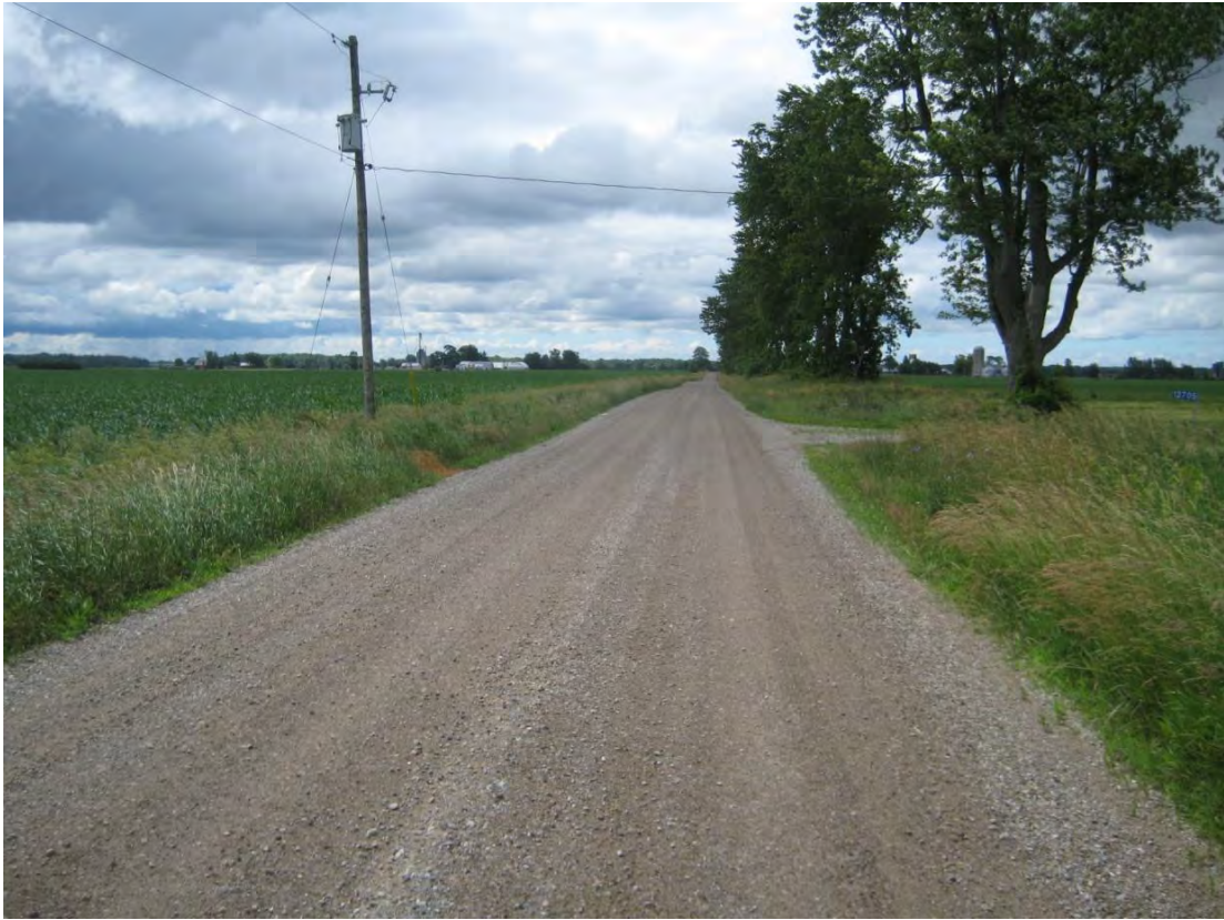
Empey Road – Inadequate road width (5.5m) with no shoulder; South of Century Line, facing South
